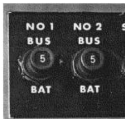
Figure 5-9 Bus Circuit Breakers
